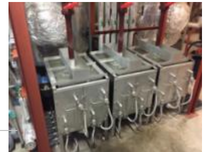
Heat exchange units
