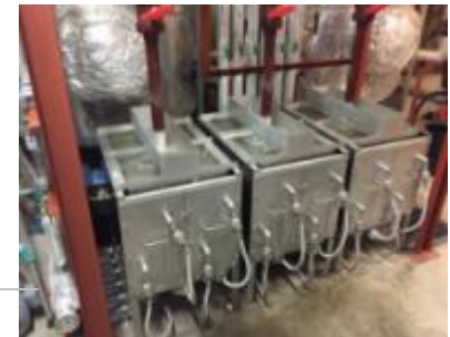
Heat exchange units
